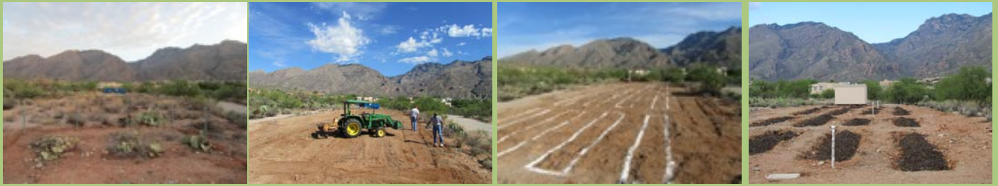
So far... site cleared, plots marked, dug, and filled with compost, shed and irrigation system installed.
